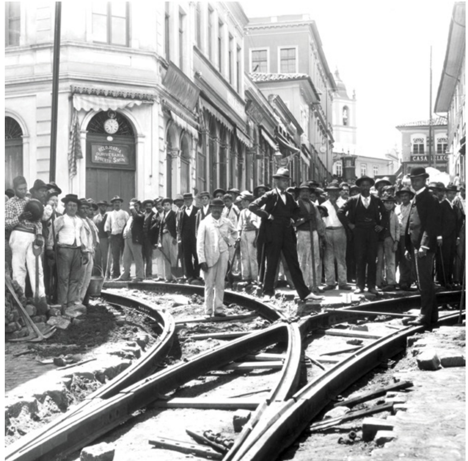
Construction of the tram line on Líbero Badaró Street, in São Paulo, circa 1900
